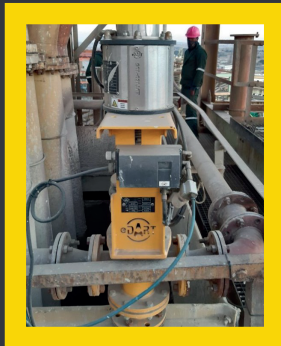
Lime Dosing Valve
